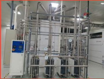
Plasma Enhanced Chemical Vapor Deposition Vacuum Pipe Line
